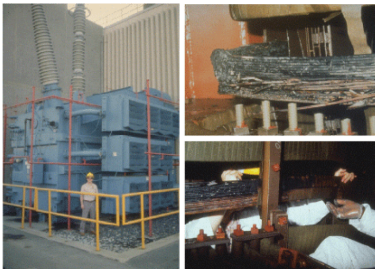
Figure 9: This is a picture of the Salem New Jersey Nuclear Plant GSU Transformer (~1200mVA, 500/22kV single phase transformer) and permanent damage caused by the March 13, 1989 Geomagnetic Storm. Photos courtesy of PSE&G.
